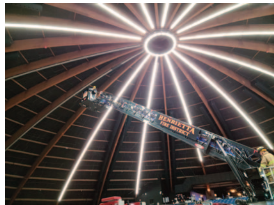
Crews respond to a ballast fire at the Dome Arena vaccine center.
