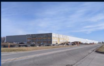
CooperVision is constructing a significant expansion, 152,950 square feet, to their facility on Thruway Park.
