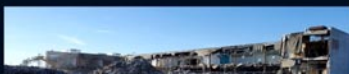
The former Macy's building at the Mall being demolished to make way for a new Floor & Décor showroom.
