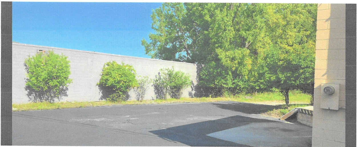
View of side of 71 Saginaw Drive building showing no Windows or doors near loading door at Saginaw Drive:
