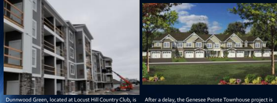
Dunwood Green, located at Locust Hill Country Club, is completing the interior of one building and starting the foundations and framing of the next.
